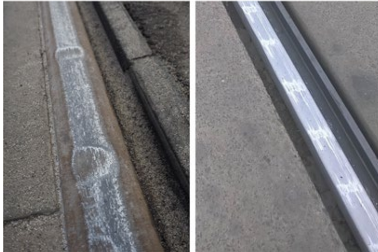
Fig. 1. Common rail defects of grooved rails
